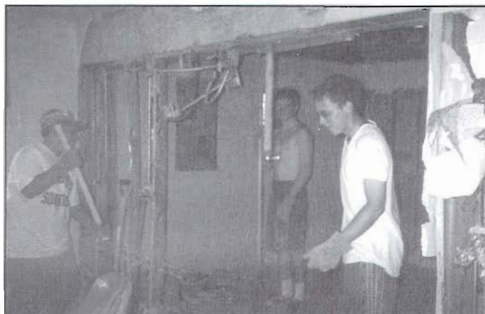
Early stages of construction of new chapter house bathrooms last summer involved gutting and completely replacing all fixtures and finishes.
